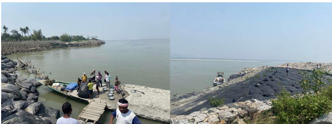
Temporary anti-erosion & flood protection works in progress by WRD/Assam Govt at Makardhuj
