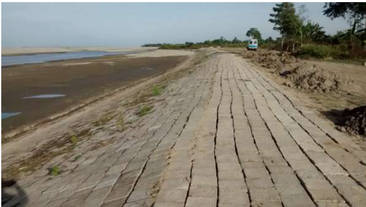
Figure 5: Typical anti-erosion work with CC block revetment and geobag apron (Motholla AE works at Motholla area by WRD)
