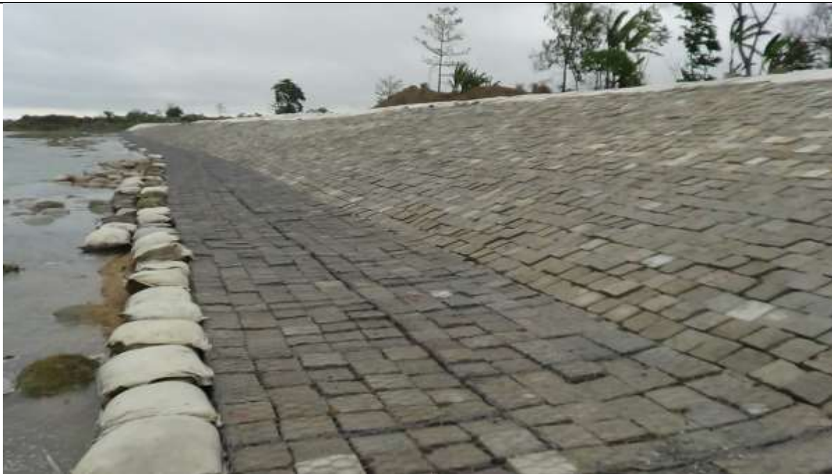
Figure 4: Typical anti-erosion work with CC block revetment and geobag apron (Motholla AE works at Motholla area by WRD)
