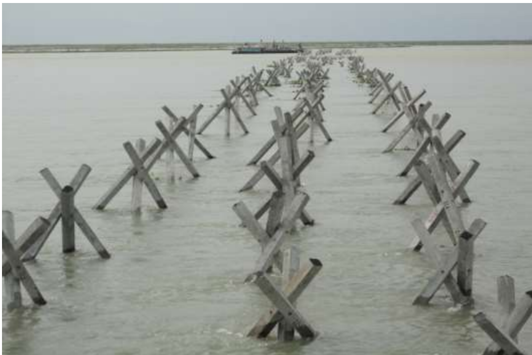
Figure 7: Typical anti-erosion work with CC block revetment and geobag apron (Motholla AE works at Motholla area by WRD)
