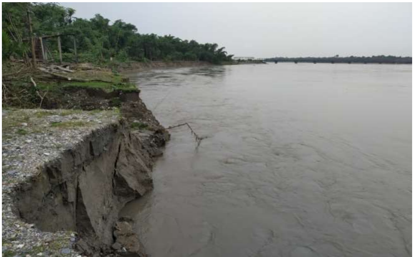
Figure 8 Erosion at Katajar
