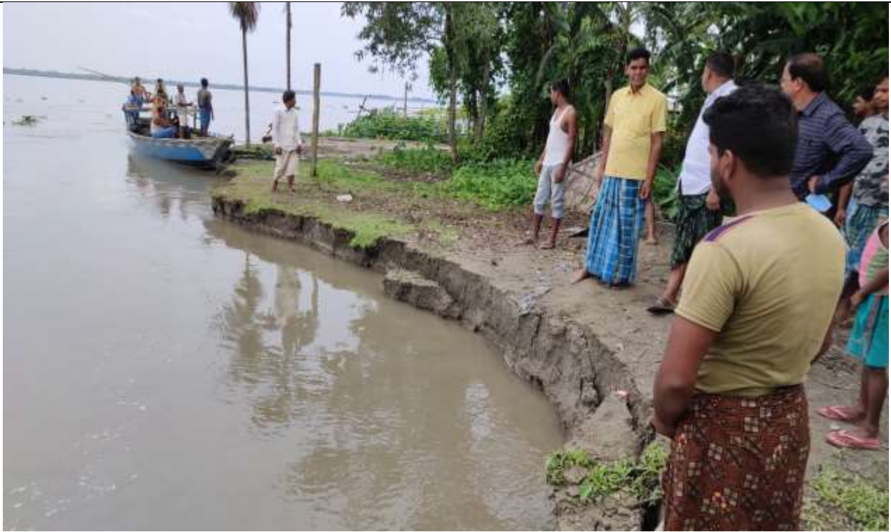
Figure 12 Erosion at Guileza
