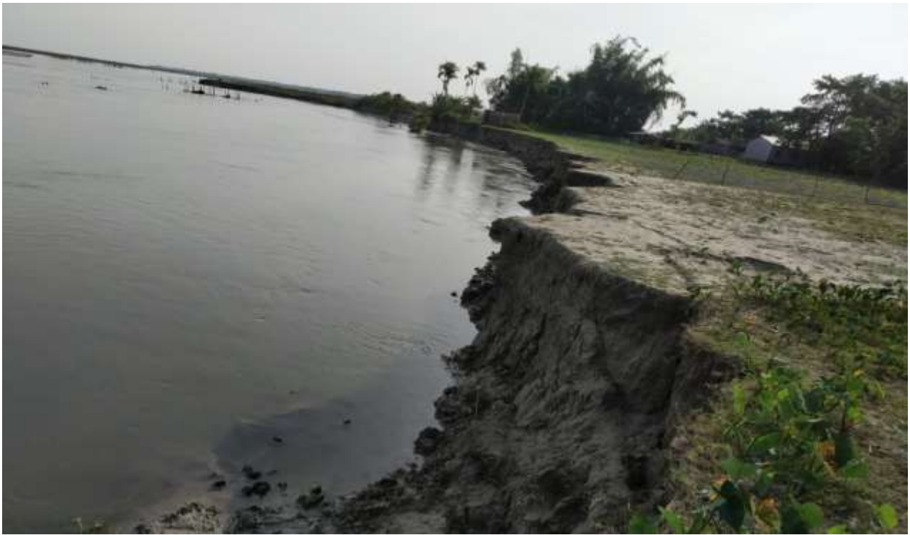
Figure 11 Erosion at Salsalia
