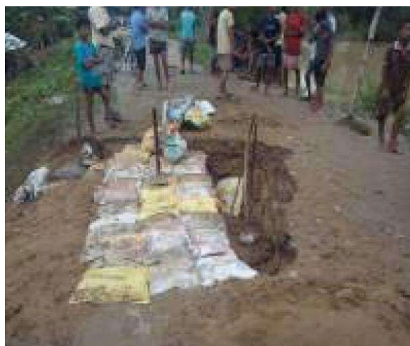
Figure 9: Current Condition of Embankment at E10
