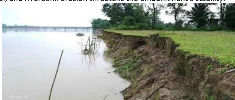
Figure 10: Riverbank erosion at Bhurbhuri-2
